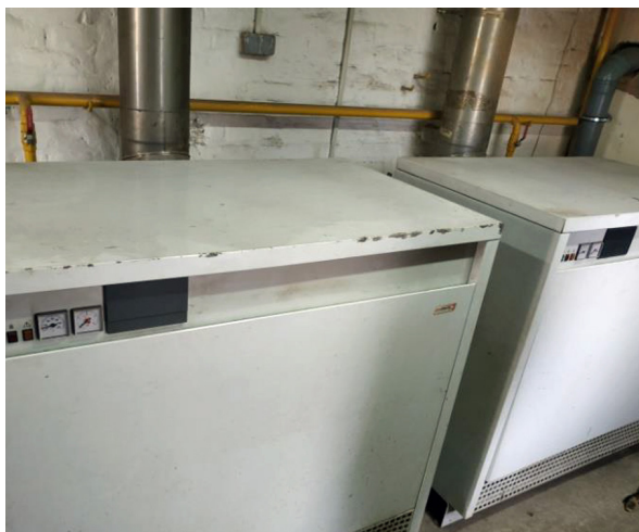
RECP recommended Olteks alternate its boiler use to optimize gas consumption.
